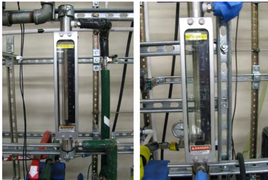
Figure C.6 Photograph of the strong and weak solution flow meters
