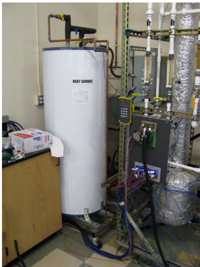
Figure 4.11 Photograph of the boiler system
